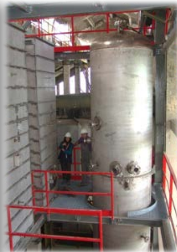
EHR pools and Drywell
