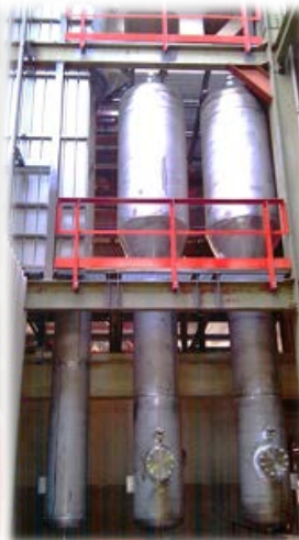
Pressure Suppression pools
